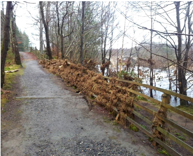
Damaged fencing at Potarch from flotsam during Storm Frank
