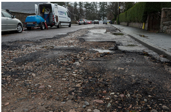
The impact of flooding on roads surface, Ballater January 2016
