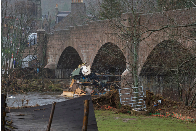
Debris build-up at Ballater bridge
