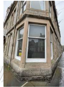
“Empty buildings are a hazard as sometimes bits fall off.”
