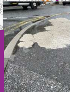
“There is damaged tactile paving across the town centre.”
