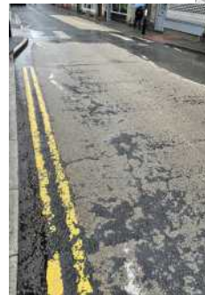
“Gordon Street – Yellow and white lines faded and the pedestrian crossing is badly faded too.”
