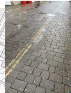
“Duke Street feels unsafe when walking with my young kids because of the lack of definition between the road and the pavement, especially when big vehicles come down.”
