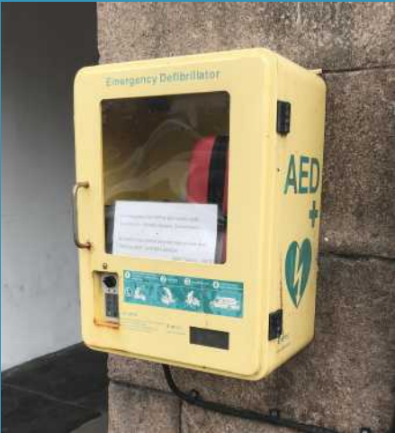
Image: Defib Unit on the side of the Market Buildings, Market Square.
