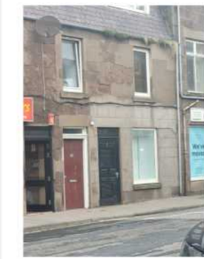
Façade needing work
