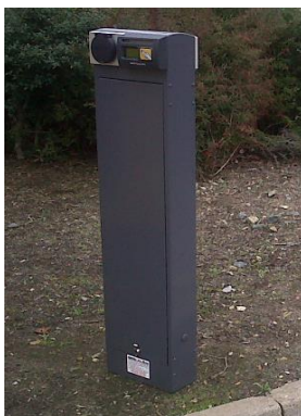
Figure 1.1: Example of a standard charging point (7kW)
